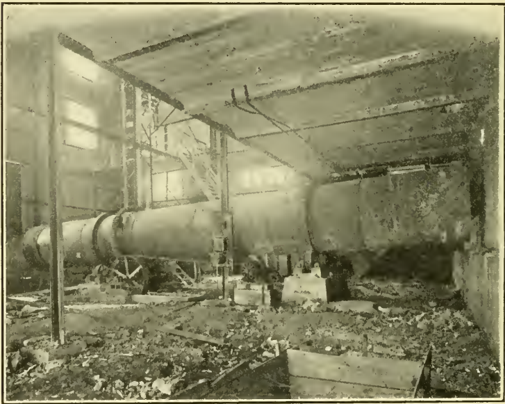
Fig. 112.—Rotary cooler—Great Western Portland Cement Co., Mildred, Kans., (Driven by Wagner Electric Co. motors.)
