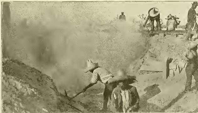
The burning of this bridge five miles from camp was reported by aeroplane and repaired reached it and started work while the bridge was still in flames. La Guna, State Chihuahua, Mexico.
