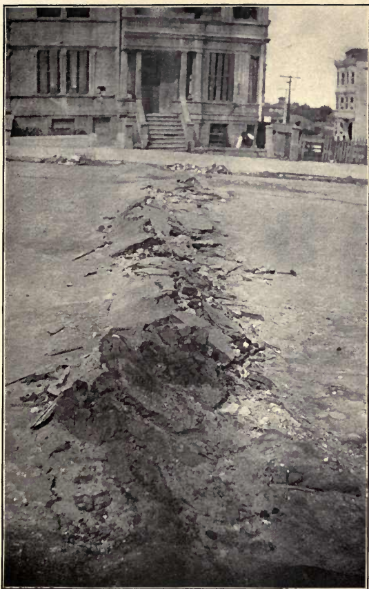
From a Stereograph, Copyright, 1906, by Underwood & Underwood A SAN FRANCISCO PAVEMENT TORN BY THE EARTHQUAKE
