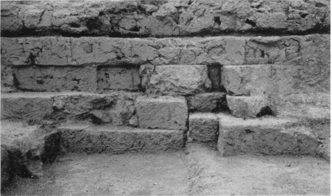
Fig. 112. Cuttings on North Side of Podium for West End of Lower Foundation and Buttress Wall
