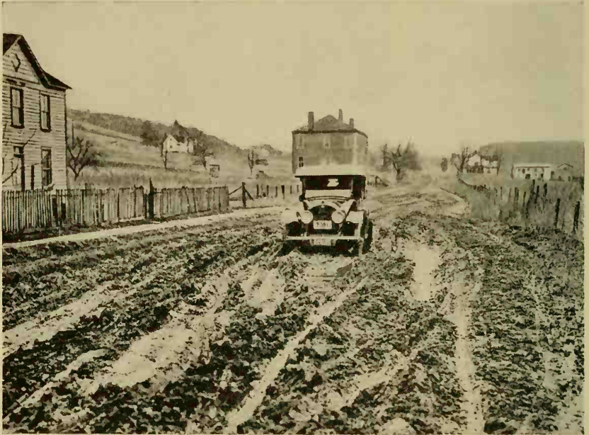
FIG. 144. U. S. 1 between Richmond and Washington in 1919. (Courtesy of the Public Roads Administration.)
