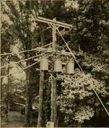
FIG. 247. Distribution transformers. (Courtesy of the Allis-Chalmers Manufacturing Company.)
