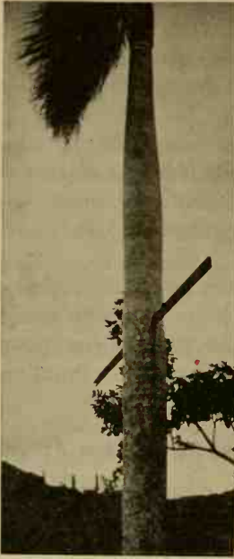
FIG. 81. Royal palm pierced by a pine board, ten feet by three inches by one inch, in the hurricane of September 13, 1928. (Courtesy of the U. S. Weather Bureau.)
